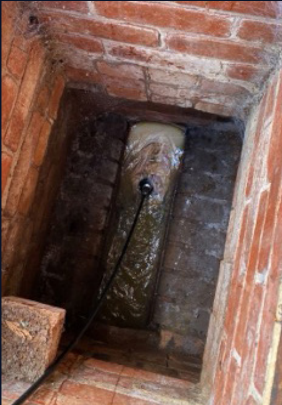
Blockage at site. Wessex Water crew successfully clear blockage before it impacts customers or the environment.
